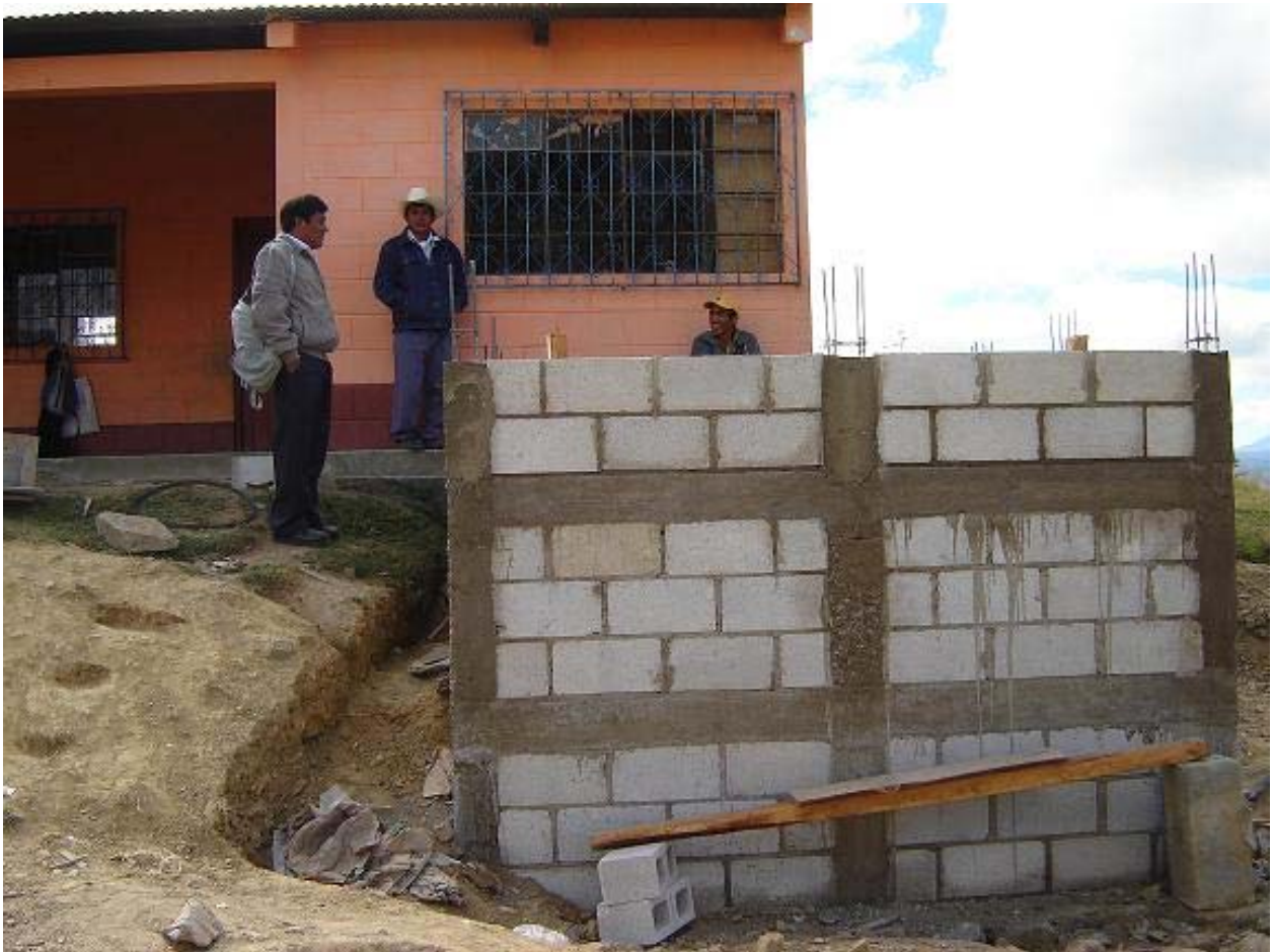
Cruz Quemada rain storage Tank
