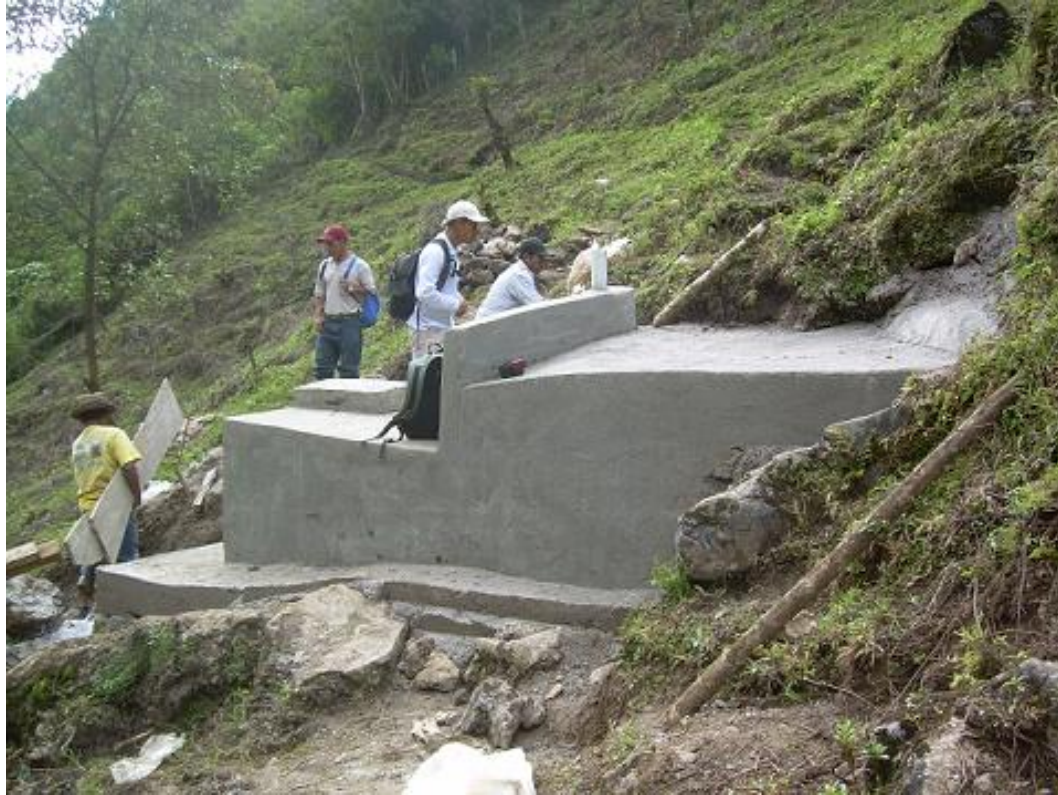
Kalampatzom spring box constructed by Juan (left) and Nicolas (right) Masons for Agua Para La Salud
