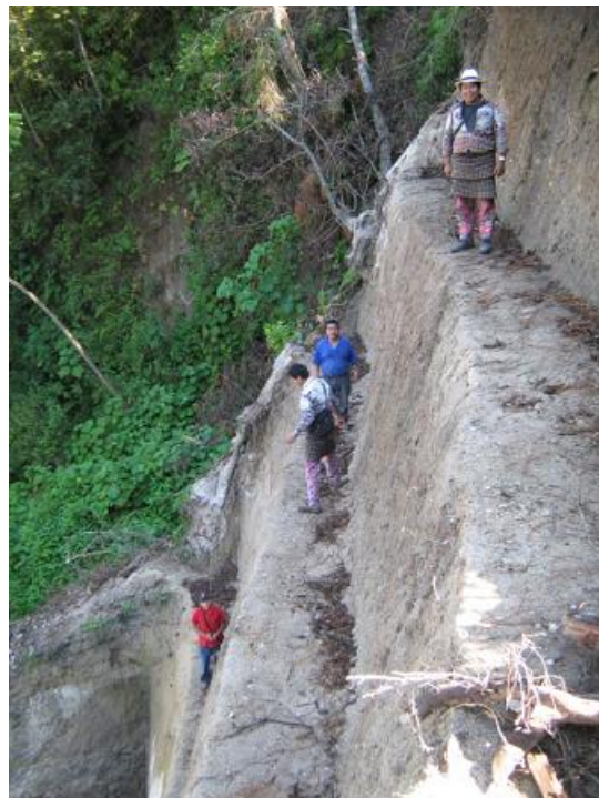
The village also spent the month terracing the hillside above the proposed tank and spring site.
